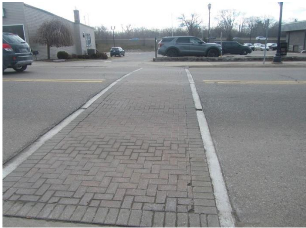
Figure 51: Crosswalk Condition Near Police Department Along Auburn
